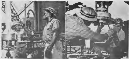
WORKMEN KEEP a careful check, above, during the operation. After the cut is completed, the plug is freed loose, right.
